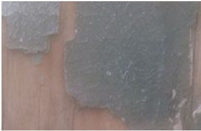
Figure 52: Peeling Paint on Door
