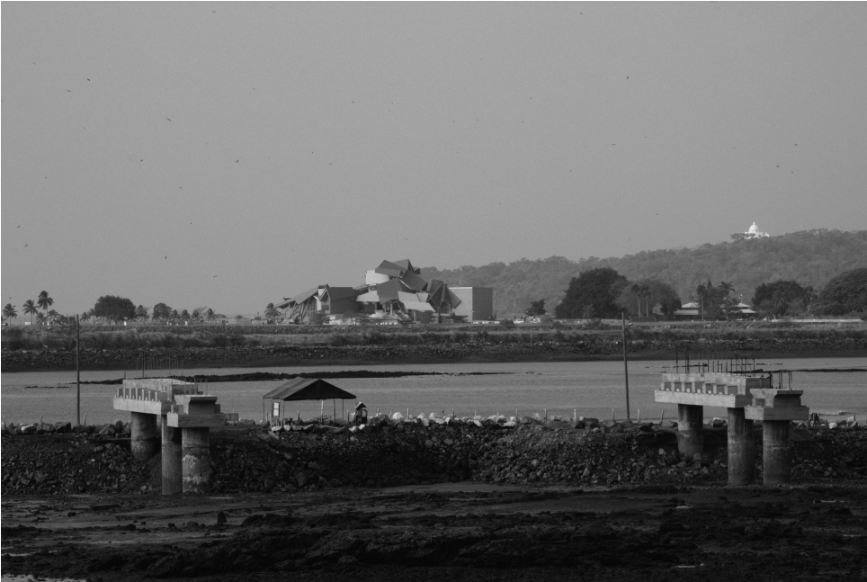
Figure 28.4 Construction of the Biomuseo from the viewpoint of la Plaza de Francia. Architect: Frank O. Gehry. Photograph by Ayaita (2013). Creative Commons Attribution-Share Alike 3.0 Unported. No changes made to image; no endorsement implied by use of this work.
