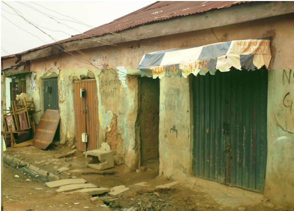
Figure 4.15: Adobe building with canopy, new doors, filled up window opening and new extension with lean-to roof at the far end
