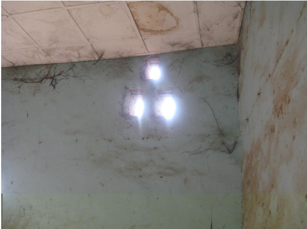
Figure 4.10: Interior of a house with leaking roof. Note the stained ceiling cause by the leakage
