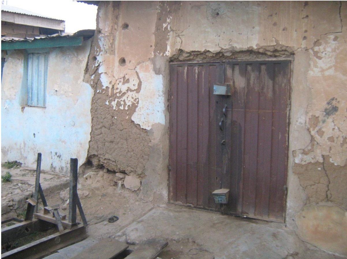
Figure 4.12: Accelerated basal erosion on adobe wall due to lack of drainage and the application of cementitious render
