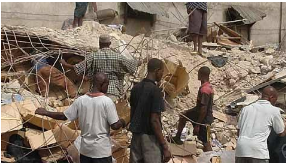
Figure 6.2: Using bare hands for rescue operation on a collapsed building site in Abuja
