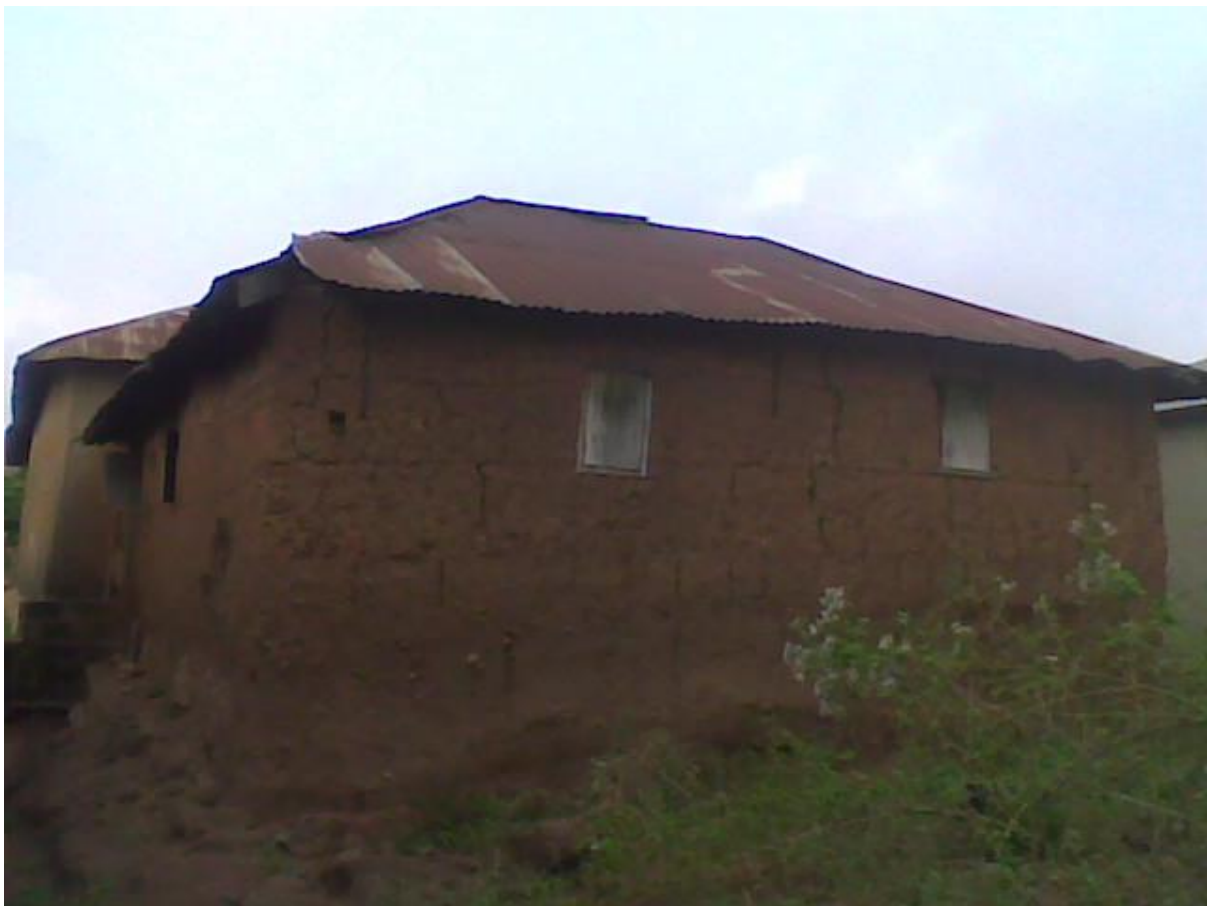
Figure 5.29 Cob buildings with cracks between lifts
