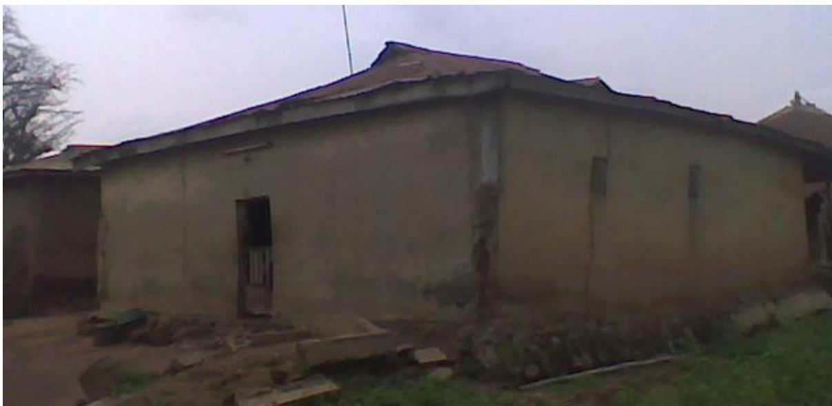
Figure 5.32: Cob building with cementitious render and stone plinth bonded with cementitious mortar
