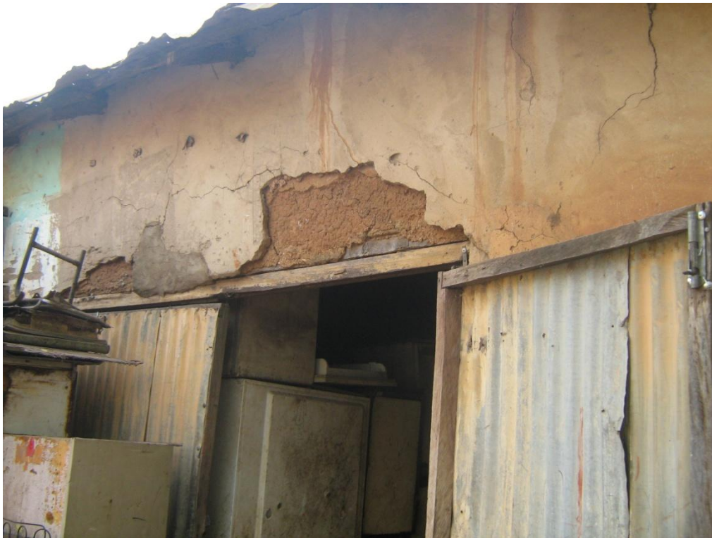
Figure 4.11: A partially deformed timber lintel caused by excessive loading. Note the cracked cementitious rendering
