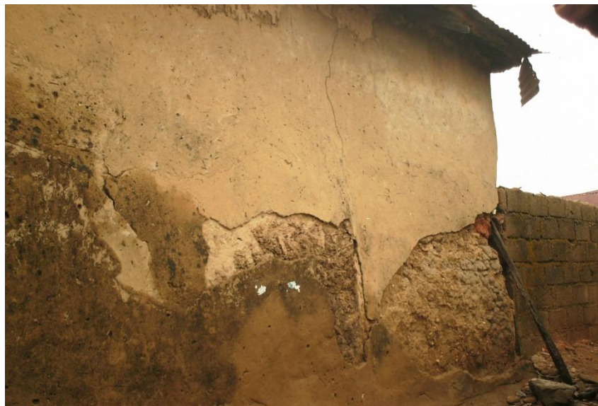
Figure 4.19: This picture is of the same building above (figure 4.16) but taken from the opposite side. The effect of rain on the adjoining property is clearer from this view
