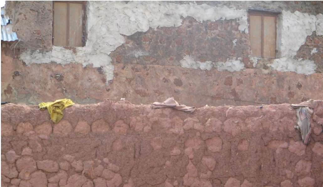
Figure 5.21: A cracked cementitious render on adobe wall
