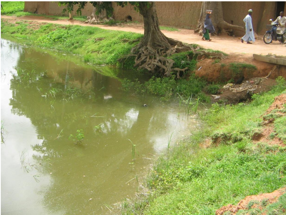
Figure 5.8: An eroded burrow pit, which is already a threat to the adjoining adobe buildings
