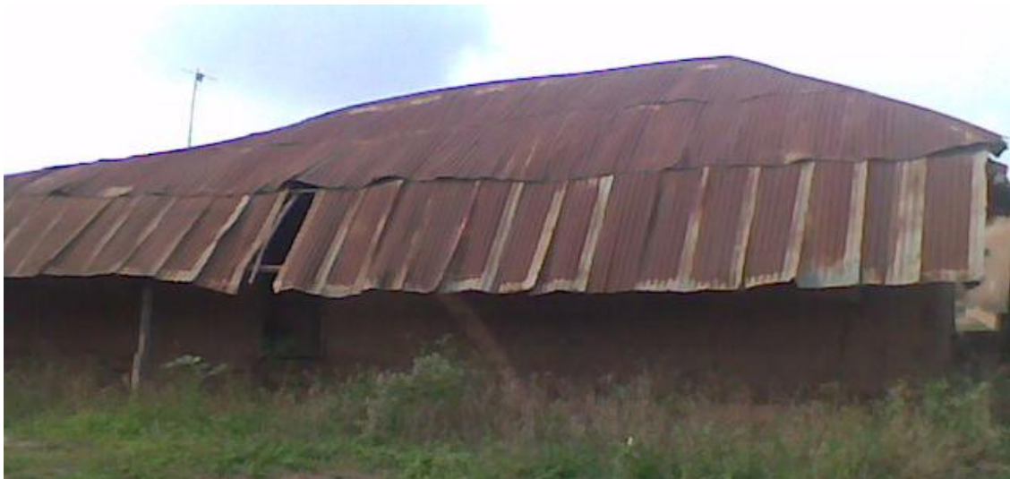
Figure 5.27: An abandoned cob building in Offa
