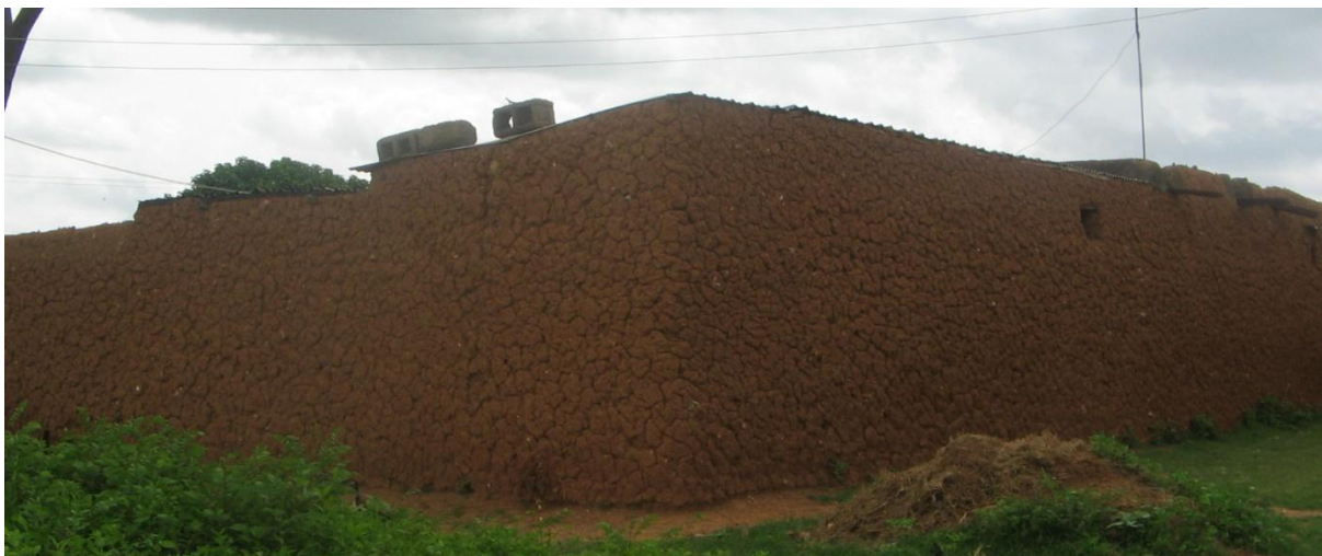
Figure 5.22: A traditional adobe building with earth based render showing minimal and even surface erosion despite the lack of roof overhang
