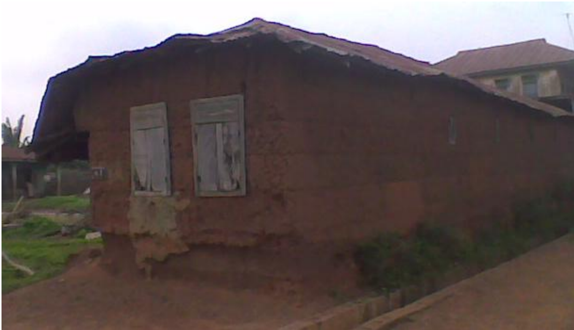
Figure 5.31: Basal erosion on a cob building in Offa
