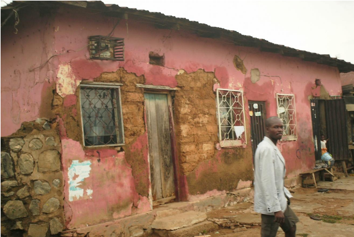
Figure 4.14: An adobe building with cementious rendering. Note the iron grills and the dampness on walls due to the rendering
